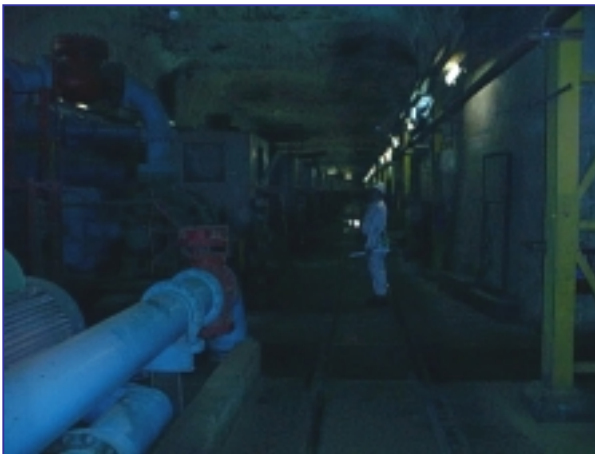
Figure 3. Pump Chamber – 985 level
